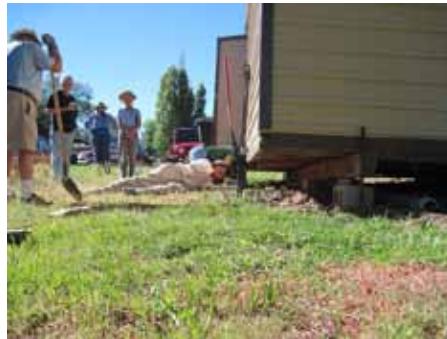
Fig. 2: Richard Stead digs out a bigger hole for a cinderblock that Paul Bradley prepares to put in place while other LAGS members look on.
